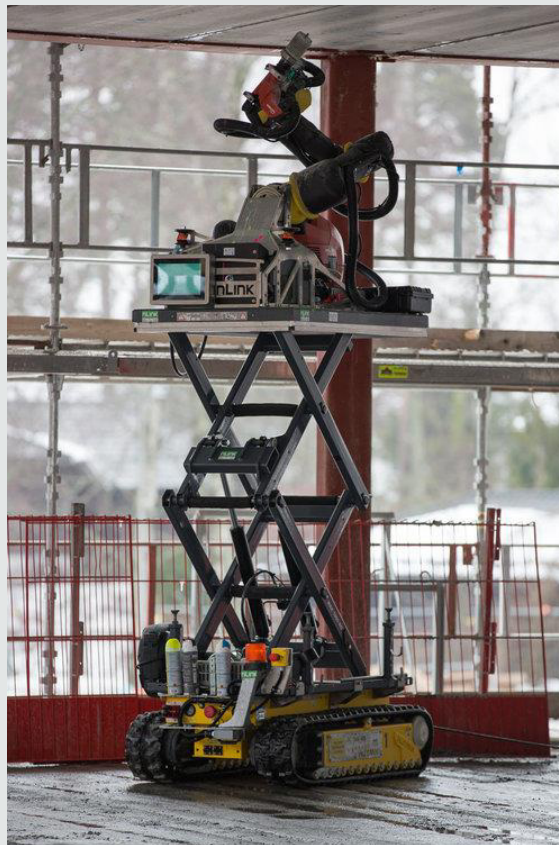
Figure 1: Examples of worldwide development on construction robots: ceiling drilling robot. Image Credit: image courtesy of nLink [20].
