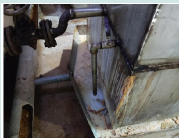
Figure 5: Leakage of waste TNT and pink wastewater from autoclave 1.
