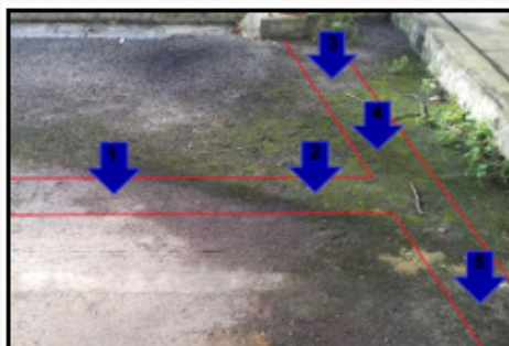
Figure 4: Wet Surface Visible at the Parking Lot Area.
