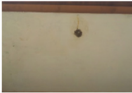
Figure 5: Watermark on the ceiling of Chancellor Building.
