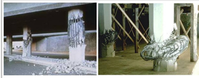
Figure 1: Failed highway bridge columns.
