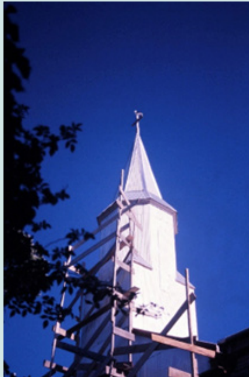
Figure 3: Chilean church being repaired (Photo taken by the author in the Chilean island of Chiloé, in 2004).
