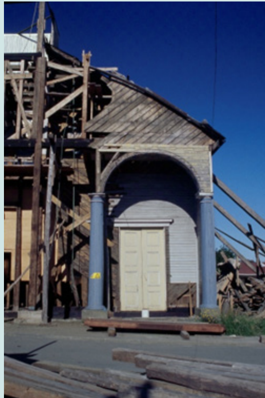
Figure 2: Chilean church being repaired (Photo taken by the author in the Chilean island of Chiloé, in 2004).
